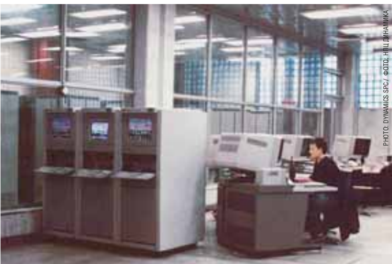
▲ The COMPACS equipment monitoring system was installed in the control room of the Omsk oil refinery's KT-1 deep refining facility in 1994.
